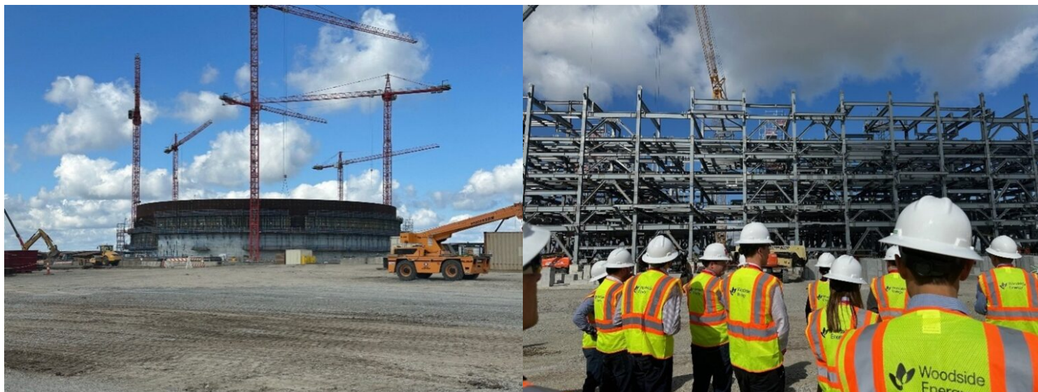
LLNG: construction of the massive storage tanks on the left, the LNG trains on the right
